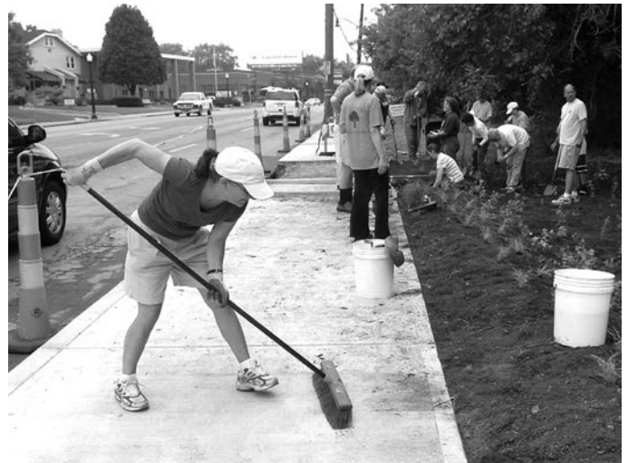
Carina Carter sweeping the sidewalk while others trim grasses between the rocks and the inlet. Approximately 33 volunteers helped install the city's first rain garden at Overbrook Drive and High Street on Saturday, September 9.
